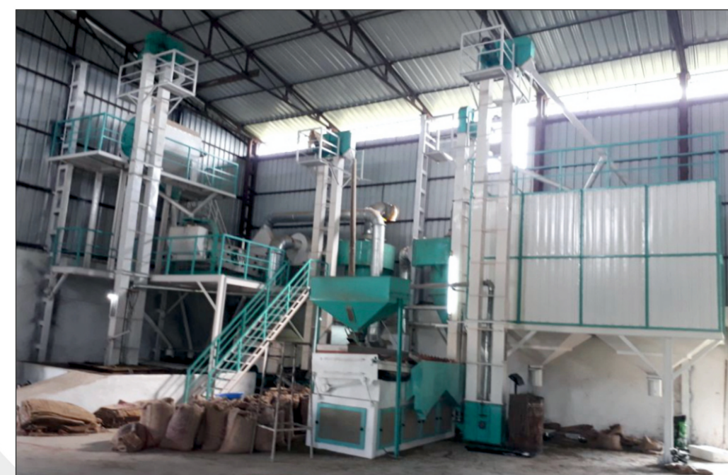
Automatic Cleaning Plant (Filter Plant)
